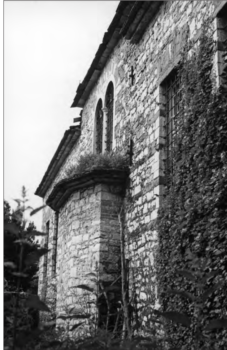
The exterior of the eastern wall of Kahal Kadosh Yashan Synagogue in Ioannina with the projection of the heikhal. (Elias V. Messinas Archive)
